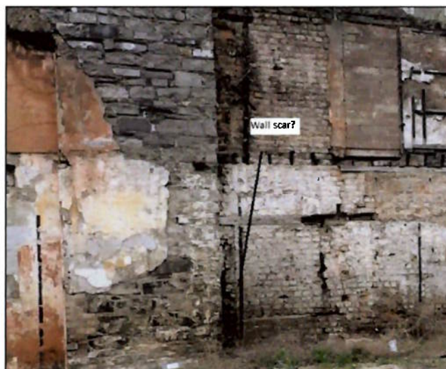
Figure 81 Wall scar of Building 2
