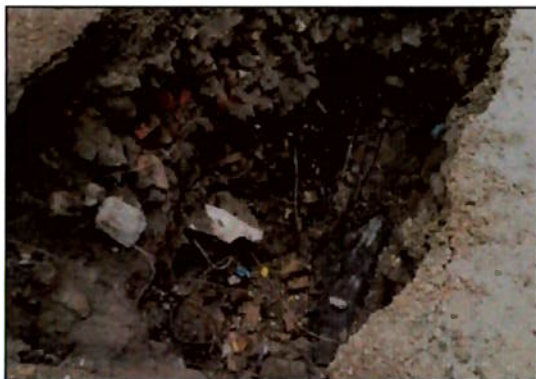
Figure 57 The floor abutting the wall foundation
